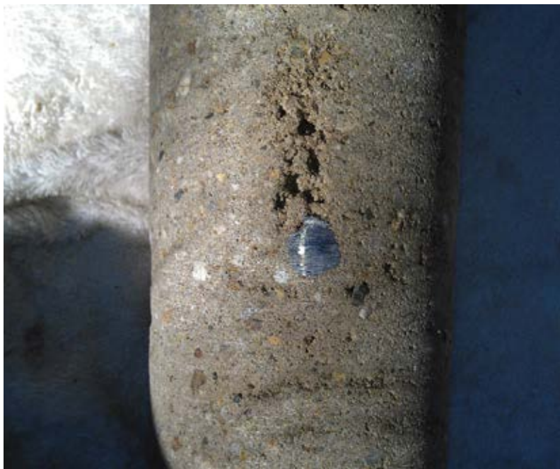
Fig. 1: Improperly compacted concrete behind steel
