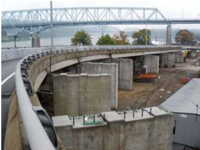
Repairs have been completed and the piers are ready for installation of the superstructure and deck in Rochester, PA
