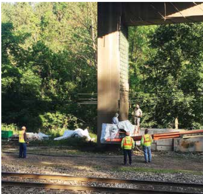
Material being cut and finished to match the original shape and profile of the pier
