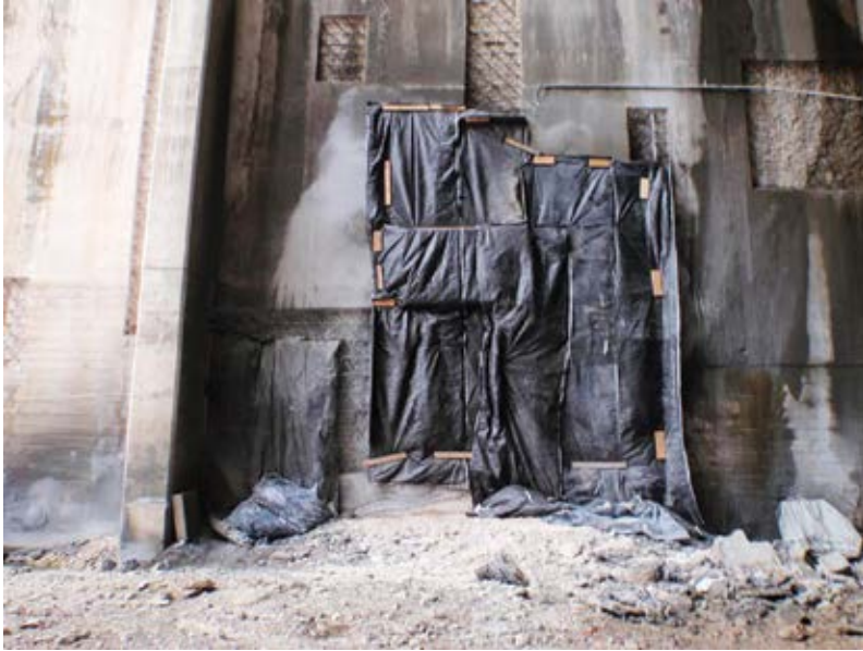
Fig. 3: Blankets and thermometers were placed on the concrete surface to monitor the temperatures through the cool night and curing period
