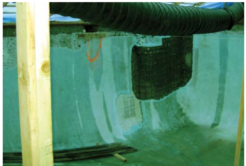
Fig. 2: High-low thermometers for monitoring the 50°F (10°C) heating within the tenting of the pool structures. The 50°F (10°C) was maintained during the shotcrete placement and curing
